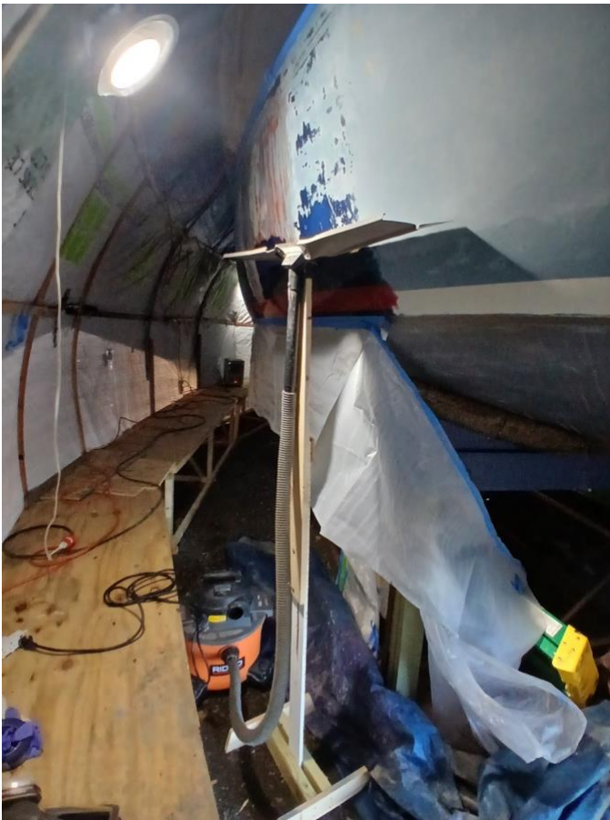
Figure 24: After stripping and scraping, the most stubborn paint would only yield to 60 grit sandpaper. Laying against the hull is a collecting tray connected to a vacuum to control dust.
