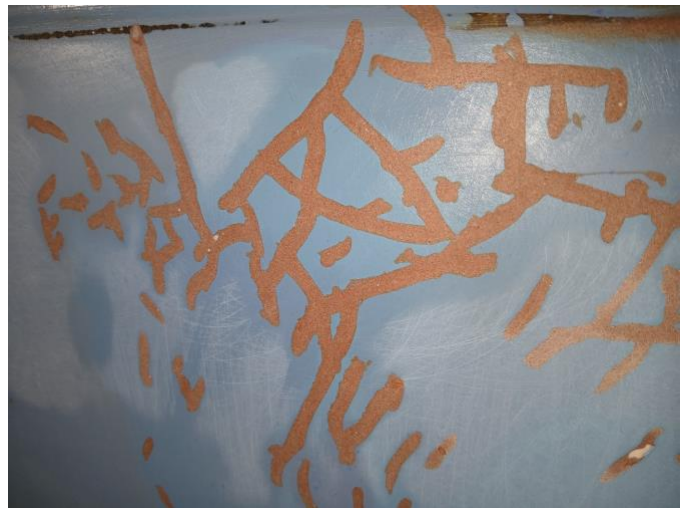
Figure 26: Hairline cracks in gelcoat, dremeled, filled, and sanded flush.
