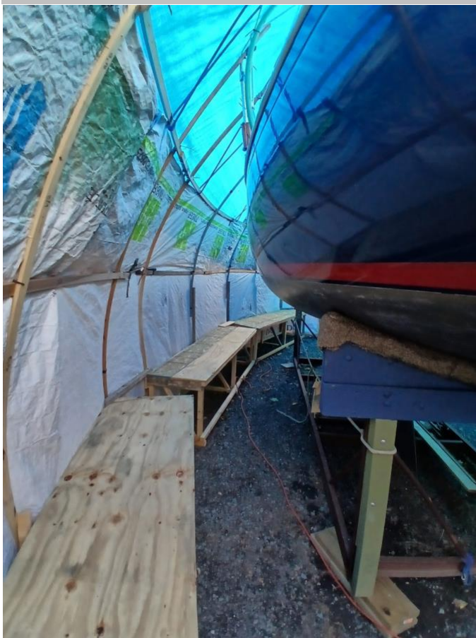
Figure 21: A weatherproof workspace and a cozy workshop for the next five months. It was dry, with electricity, lighting, and even piped-in hot air during the coldest months.
