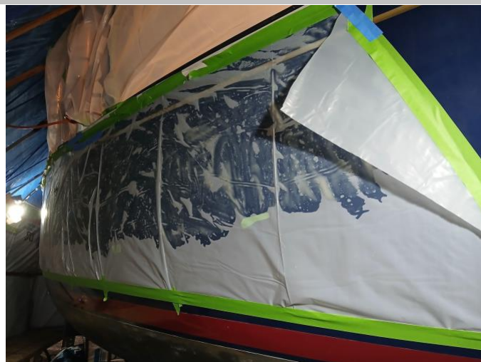
Figure 22: The stripper doing its work. The key was keeping it damp (covered) and working in sections.
