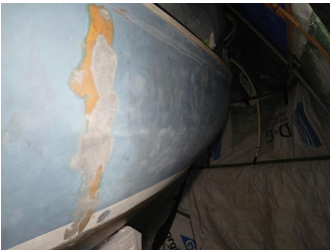
Figure 25: Evidence of a previous attempt to repair. Gelcoat burned away by a previous effort.
