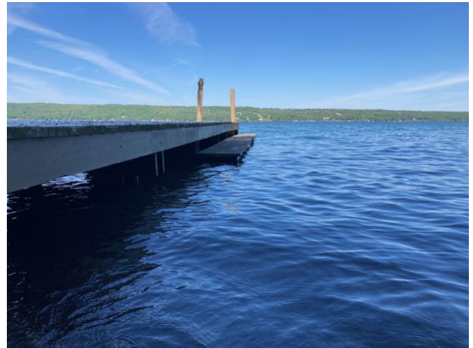
Figure 1: Side dock revealing approx. 4" drop as of 5/26/26.
