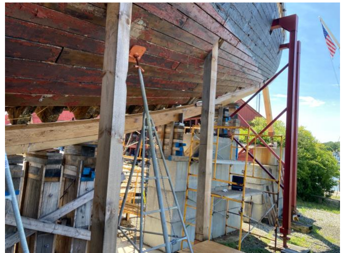
Figure 2: Mystic Seaport boat support system penetrating the boat.
