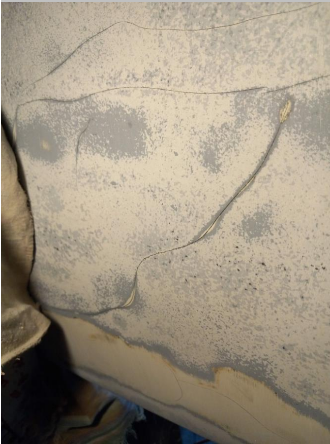
Figure 5: Hairline cracks below the waterline.
