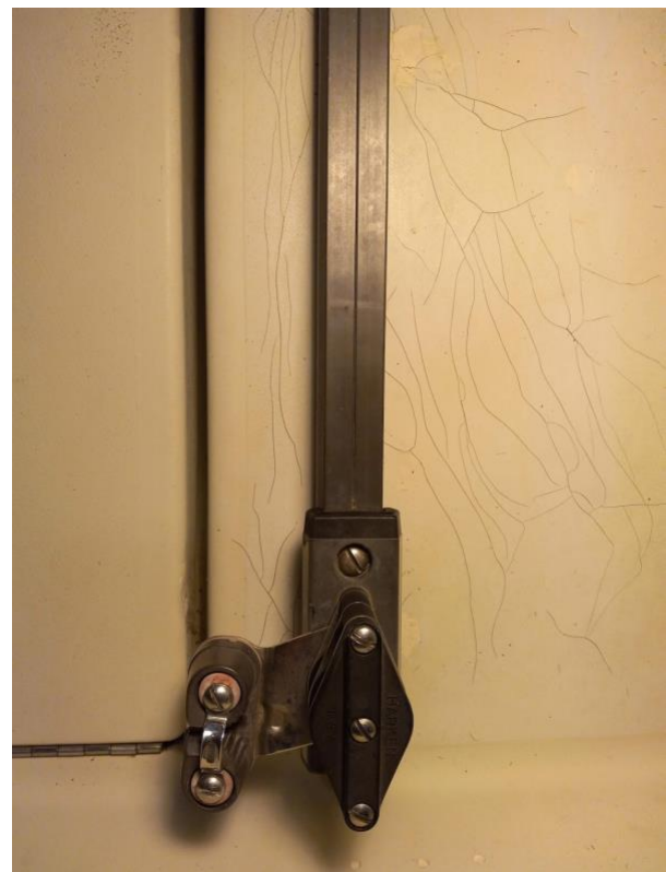
Figure 2: The "blemish" on the starboard side of the bridge deck. This was taken at the end of 2022 season but had not changed much since taking ownership in 2017.
